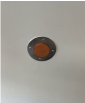
Hole for cable inlet
